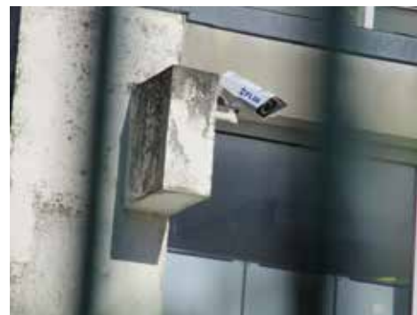
The camera has been installed on the roof of an adjacent building without the use of a mast.
